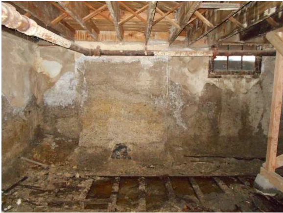
Photo 13: Southwest corner of basement has standing water and rotted earth supported floor joists. A temporary support is at the right of the photo.
