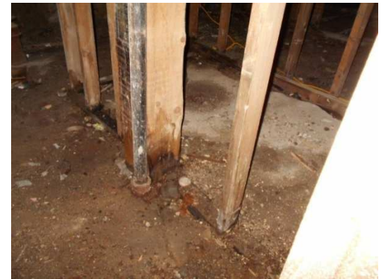
Photo 12: Water damage and rot where columns and wood walls are in contact with dirt basement floor.
