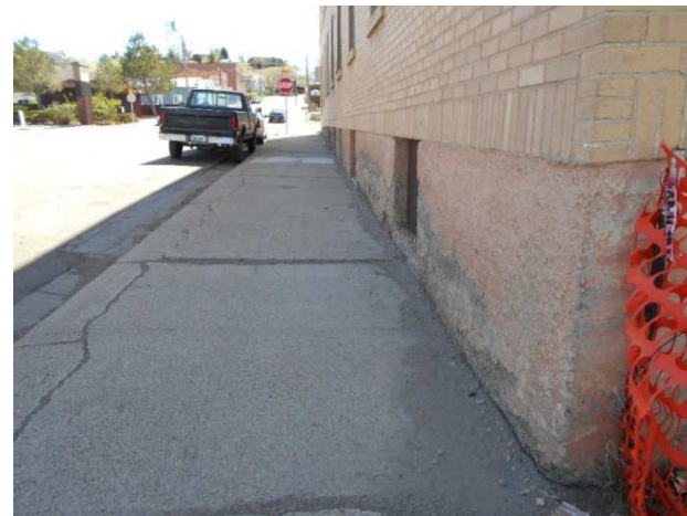
Photo 22: Sidewalk at east wall slopes toward the building.
