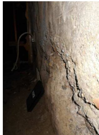
Photo 16: Looking south along deteriorated section of west basement wall.
