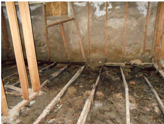
Photo 14: East wall of basement with wet soils and rotted floor joists.
